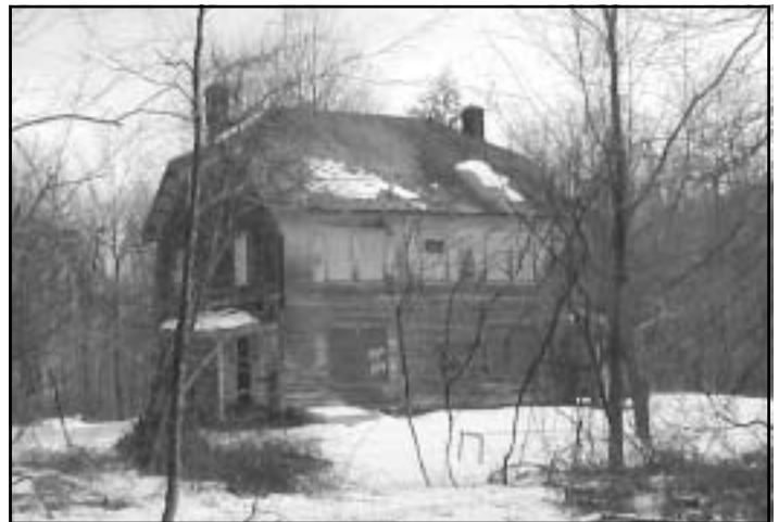
Recent view of the back of the Manager's House. This building and the industrial remains in the Furnace Area are considered the most important structures for preservation at Long Pond.
